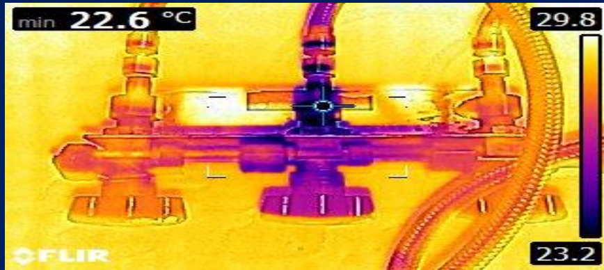
INFRARED THERMAL IMAGE
