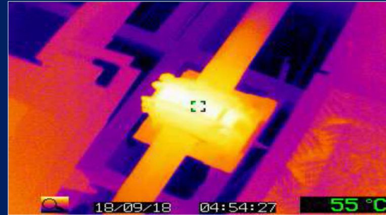
THERMAL IMAGE OF SHAFT BEARING
