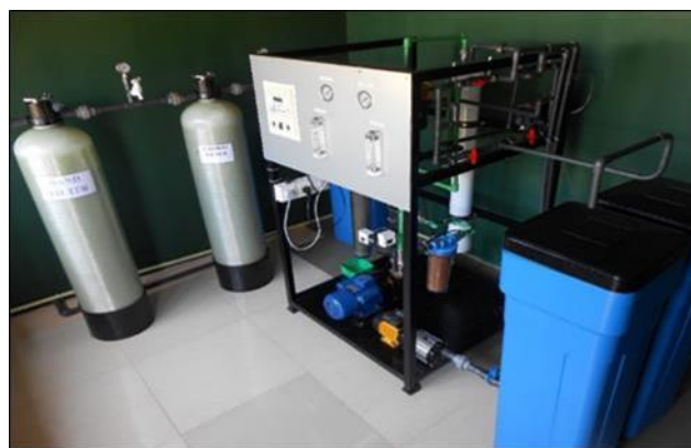
Figure 2. The Brackish Water Reverse Osmosis Plant with a capacity of 10 tons/ day was developed by Sri Lanka Navy.
