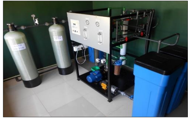
Figure 2: Capacity of 10 Tons/day, brackish water reverse osmosis plant developed by Sri Lanka Navy
