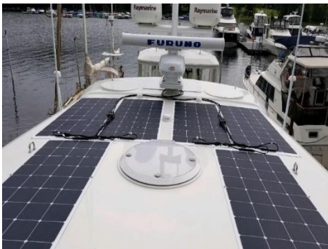
Fig 4. Flexible Solar Panels
